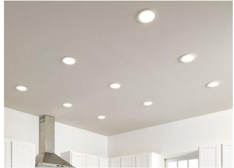
Structured Indoor Lighting 1
